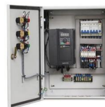
VFD Panels integrated with MCB, On-off switch, potentiometer, Push button, etc.
