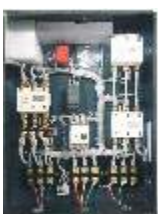
Interior View of MU-G30W FASD
