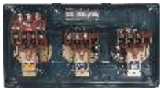
Interior View of MK2 SASD
