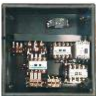
Interior View of MU-G20W FASD
