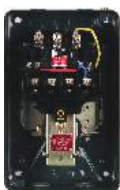
Interior View of MK1 DOL
